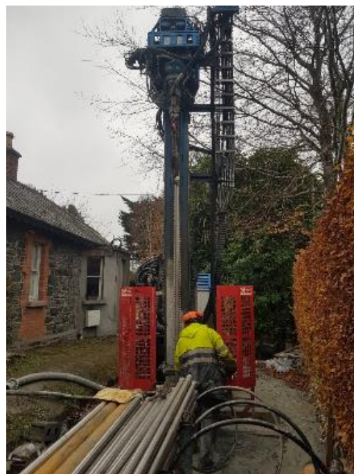
Installation of the heat exchanger
