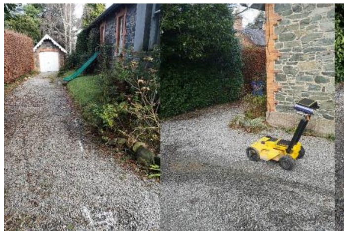
Figure 8 GPR surveying at the Greystones case study site in Ireland to map the location of services and structures.
