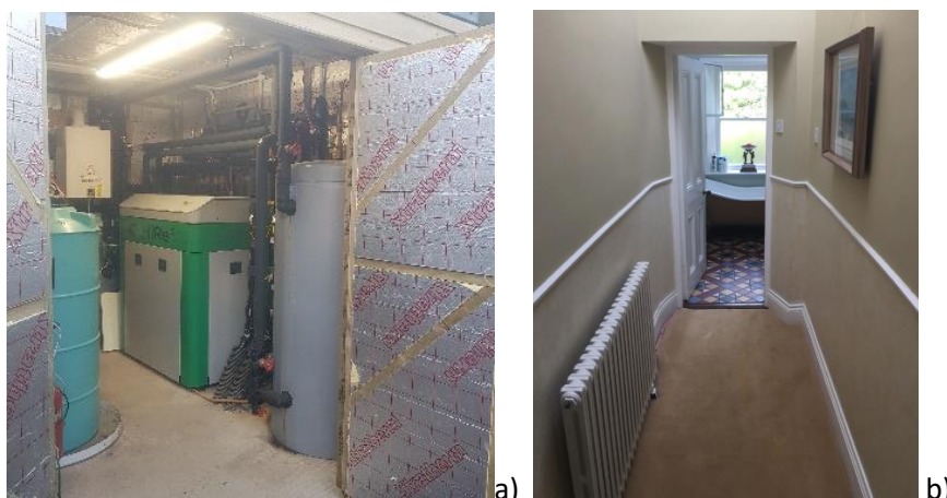
Figure 4 Ireland case study site showing a) external plant room and b) integration of the GSHP solution to existing high temperature radiators
