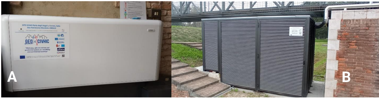
Figure 6: Fan coil (A) and technical room (B) (Finotti copyrights)
