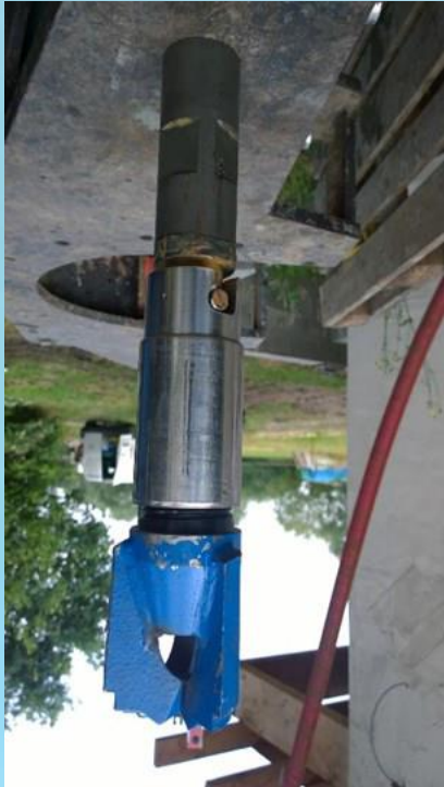
drill bit entrained by the shaft
