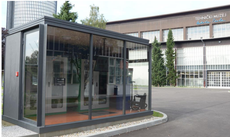
Figure 1. High temperature cascade cycled heat pump installed at the Tesla Technical Museum in Zagreb (Croatia)
