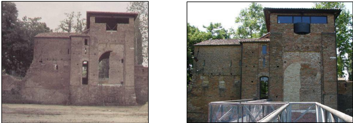
Figure 5 - Before and after restoration work on north archway and closing of it
